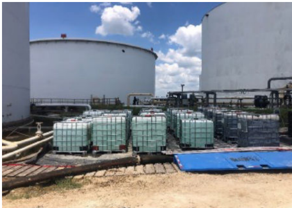
Totes of ThunderOx chemistry and oxidate on site at the refinery
